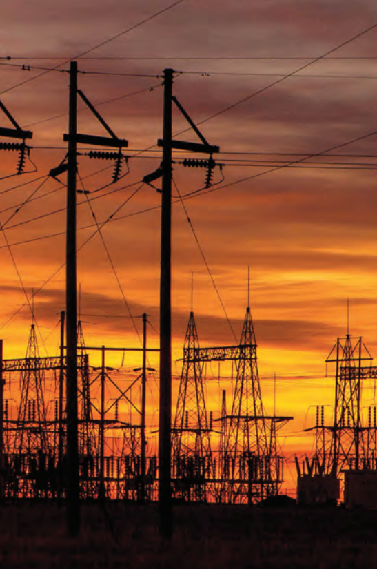
A complex web of high-voltage power lines and power plants deliver electricity across millions of miles of lower-voltage lines connected to energy consumers. PHOTO BY JAMIE FOWLER, HIGH WEST ENERGY INC.
