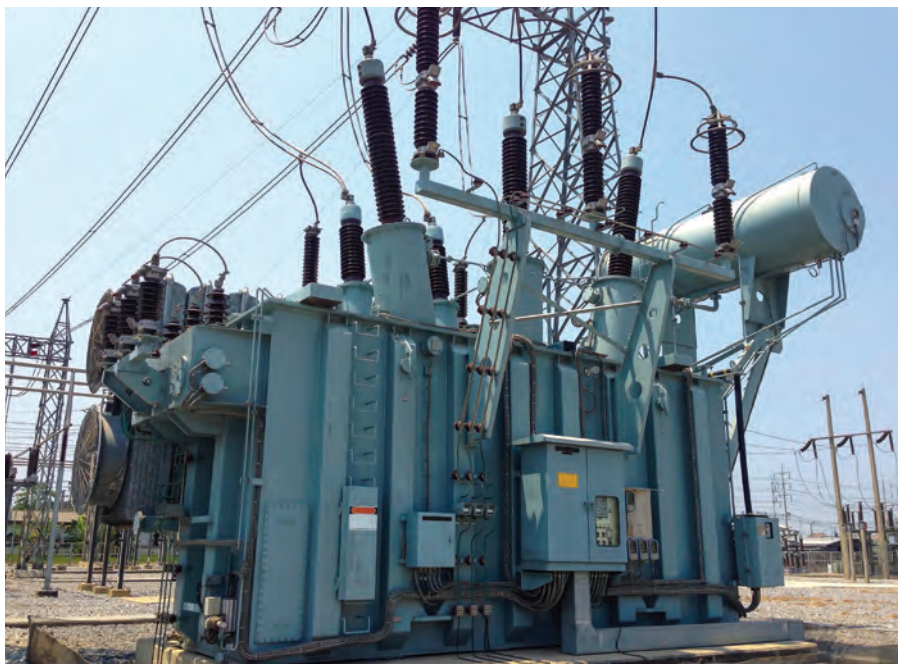
Transformers are a hot commodity for electric utilities. Steel shortages, coupled with a lack of manufacturing workers, mean transformer manufacturers are unable to keep pace with a significant increase in demand. ADOBE STOCK PHOTO BY CHII CHOBITS
