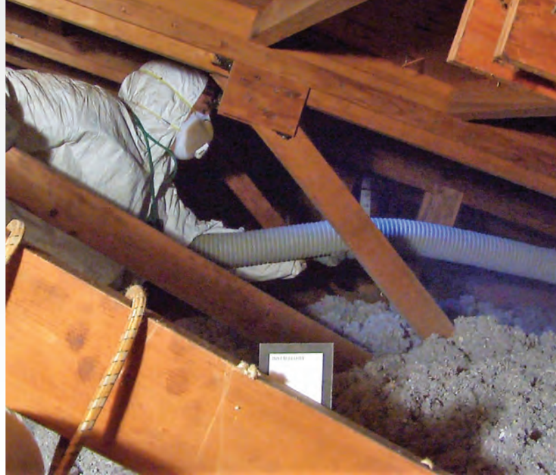
A contractor installs blown cellulose insulation in an attic to minimize energy waste. PHOTO COURTESY OF PROJECT HOME
